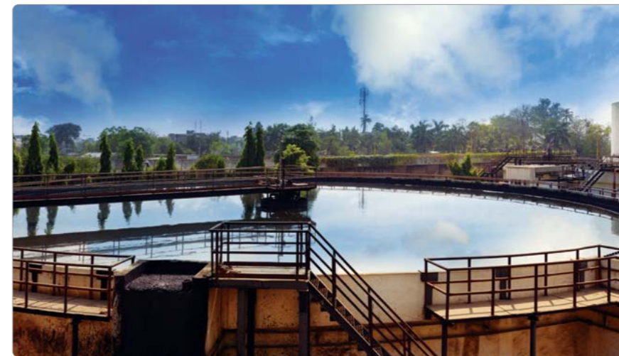
Clarifier at Gujarat Refinery for treatment of sewage waste for reusing water
