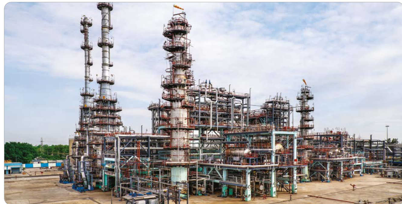
▶ A Process Unit at IndianOil Gujarat Refinery
