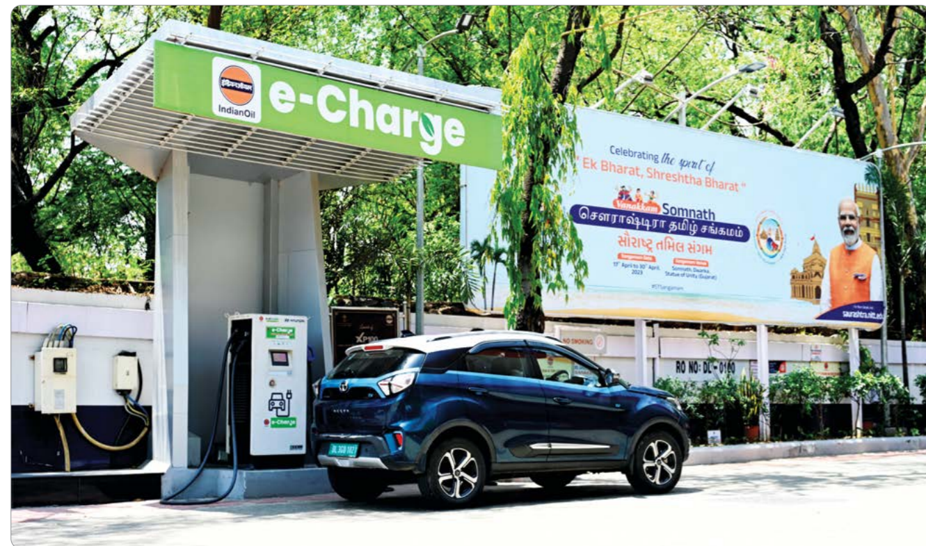
EV Charging Facility at IndianOil fuel station
