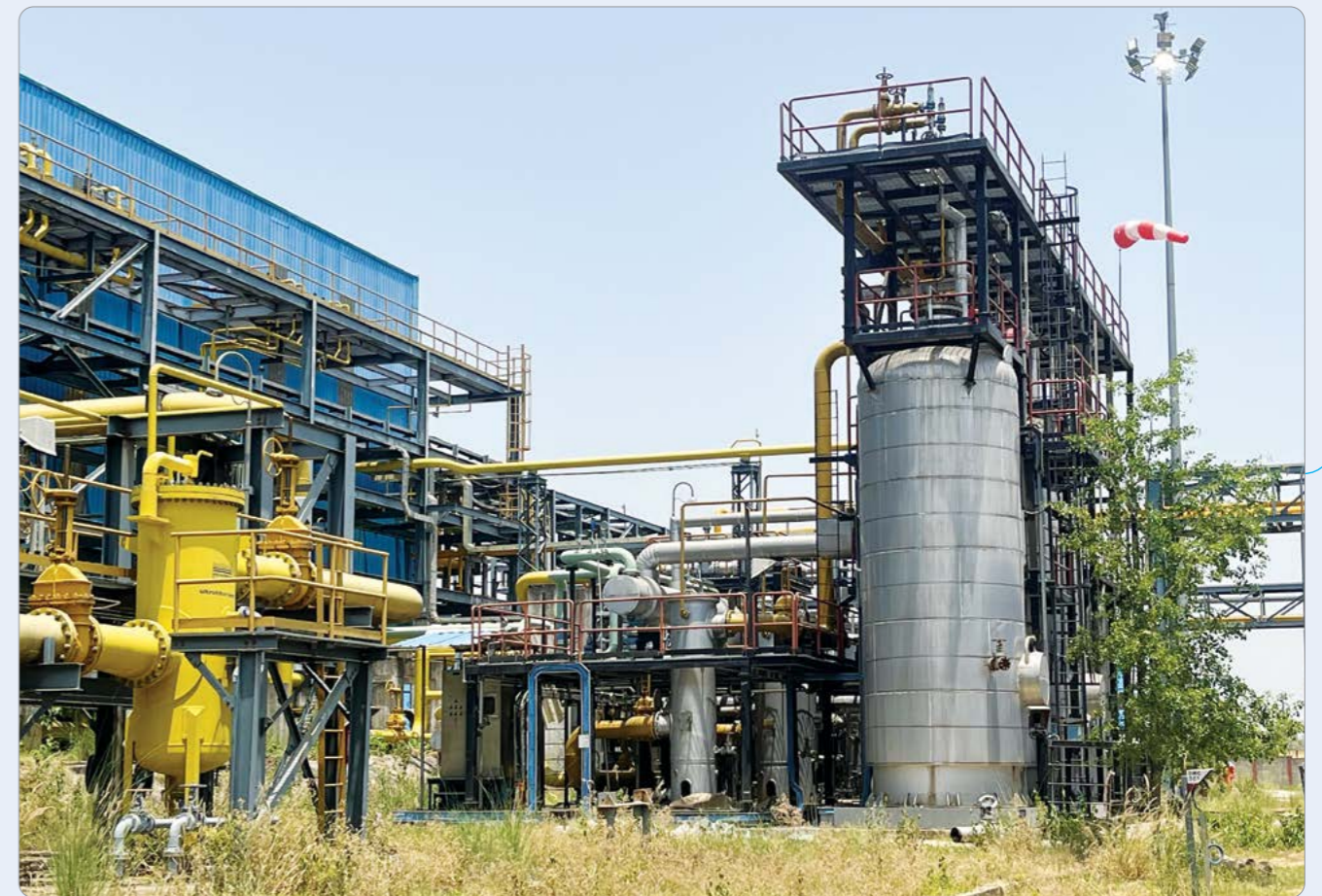
Gas Collecting Station (GCS), Bokaro- a major production installation for processing of Coal Bed Methane gas
