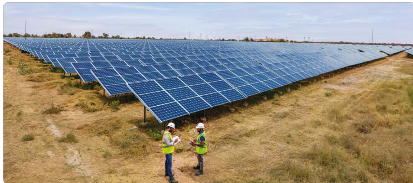
IndianOil Rawra Solar Power Project in Rajasthan
